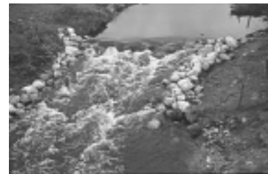
Seek expert advice if installing bed control structures such as rock chutes
